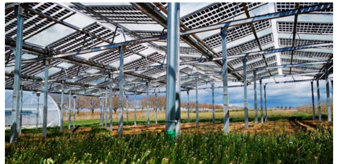
Figure 3: Sample use of semi-transparent PV panels by MKG Göbel
